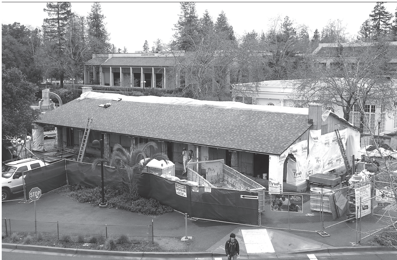
East Cottage with half a roof in March 2011. It is now wholly roofed. Photograph by Purba Fernandez.
